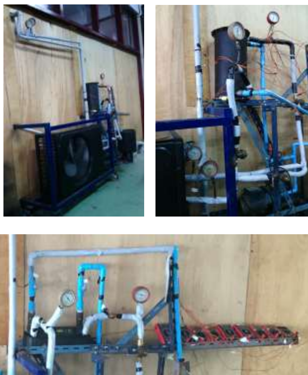
Fig.3. Condensing Unit, Pressure gage, Control Valve and Hot Water Tank
